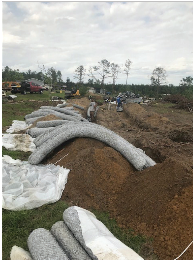
Installation of a new septic system for one of the Disaster Relief families in Lee County.
