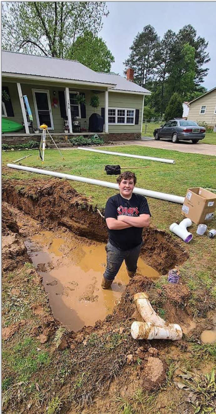
In the trench shooting grades is one of C.J. Gulley's favorite places to be at an installation work site.
